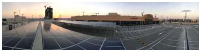
Enerwhere solar installations at MyCityCentre Al Barsha
